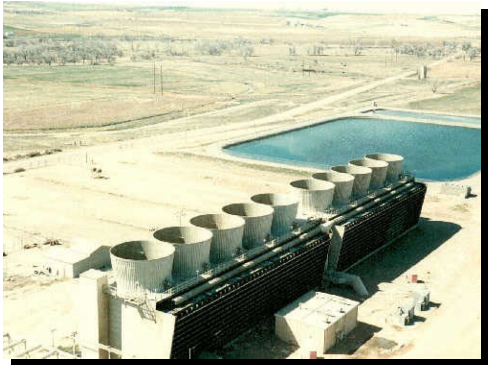
Power plant cooling tower.
