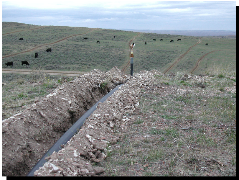
CBM water is piped to fields to be used for irrigation in this solid-set system. Note the use of "water cannons" attached to the PVC pipe. This method of irrigation has proved to be very cost-effective.
